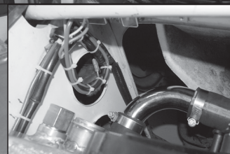
Left and above: The simple added wiring for the fans was run along the bottom and up the side of the internal sheet metal to the controller.
